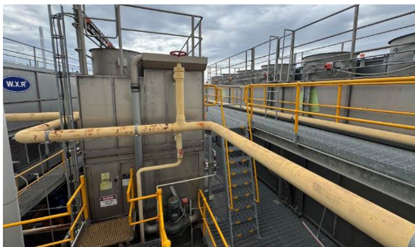
Figure 2: View of three (3) of the five (5) WXR2000 cooling towers.
