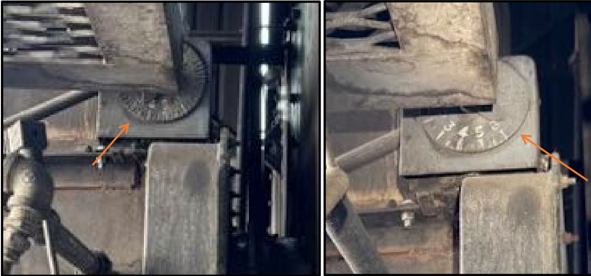
Figure 12: close up of the bed height manual controller indicator (left) set at ~3.5" for coal; (right) set at 6.5" for the pellet/coal mix.
