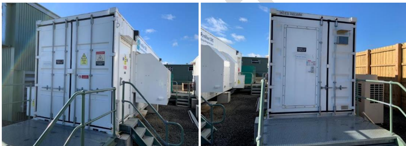
Figure 38. Behind-the-meter BESS installed for Hardwicks of Kyneton microgrid
