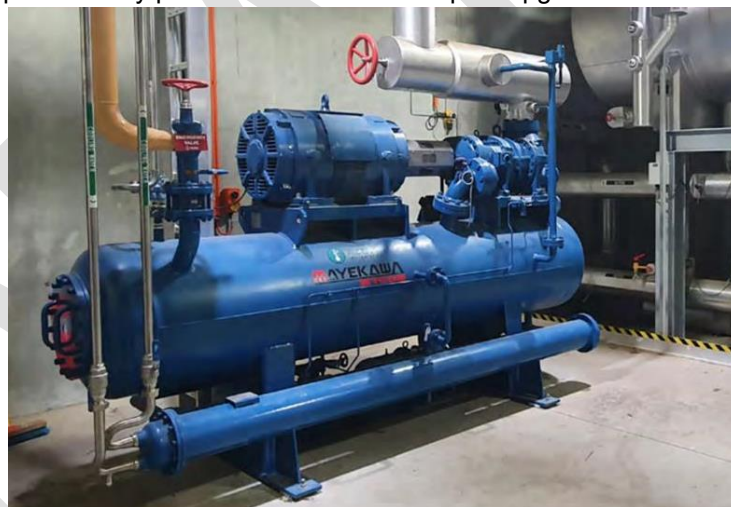
Figure 31: Mayekawa 90°C Water to Water Heat Pump installed in Food Industry (DETA).
