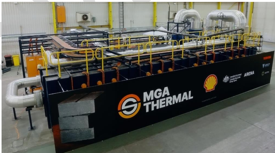
Figure 33: MGA thermal's ETES demonstration plant (MGA Thermal, 2024)
