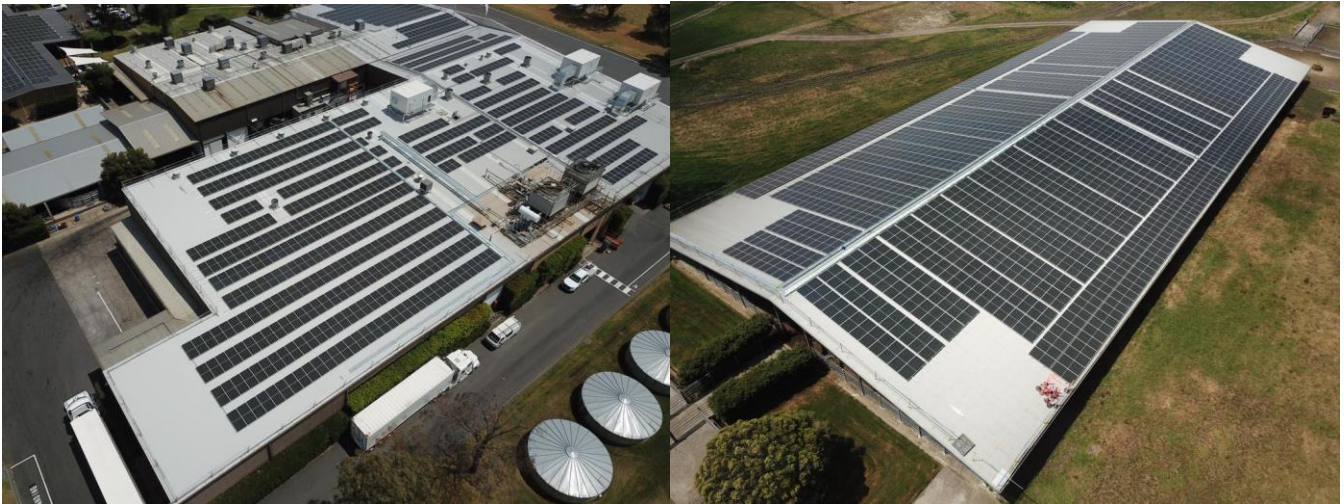
Figure 36. Rooftop PV System installed at G & K O'Connor abattoir in Pakenham, Victoria
