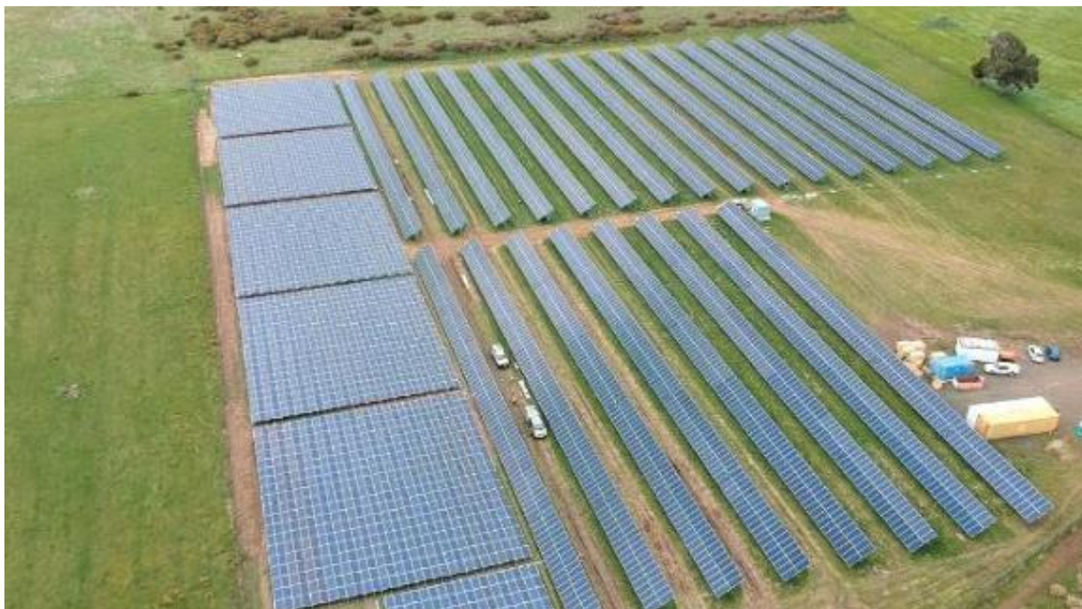
Figure 37. Ground-mount solar array installed for Hardwicks of Kyneton microgrid
