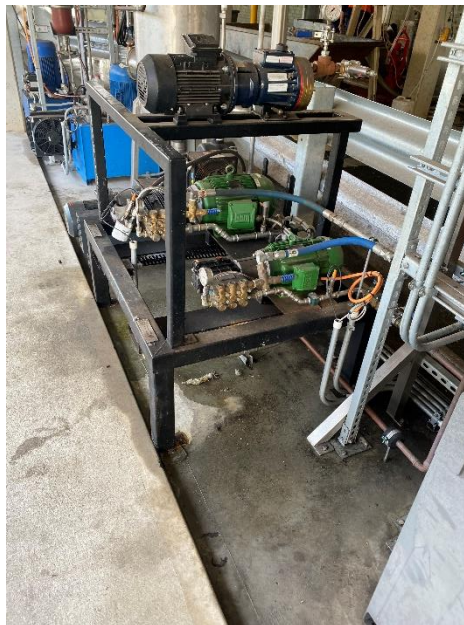
Image 2: OEM and Warble Pump Station
