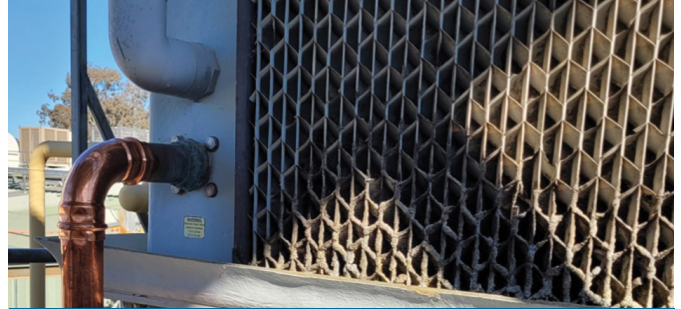
Figure 6 Engineering controls on condenser – RPZ and air gap.
