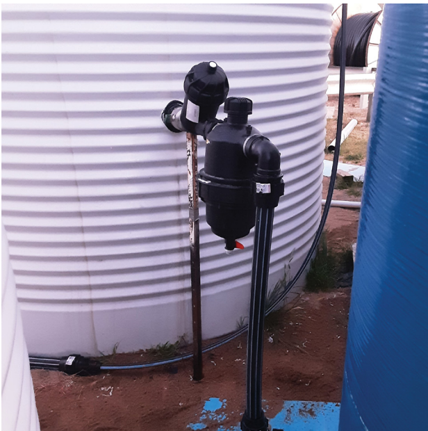
Figure 2 Tank “clarifier” and screen filter.
