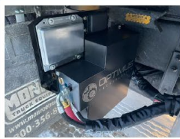
Installed Vector Manifold and ECU
