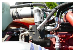
Automated Fuel Selector Valves
