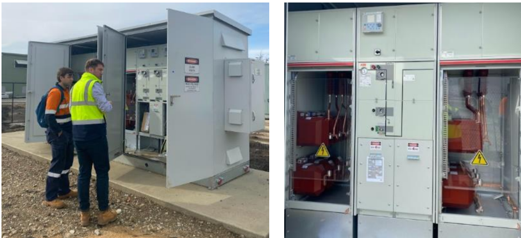
Figure 26: New 22kV switchboard (High Voltage) due to be commissioned in December 2022
