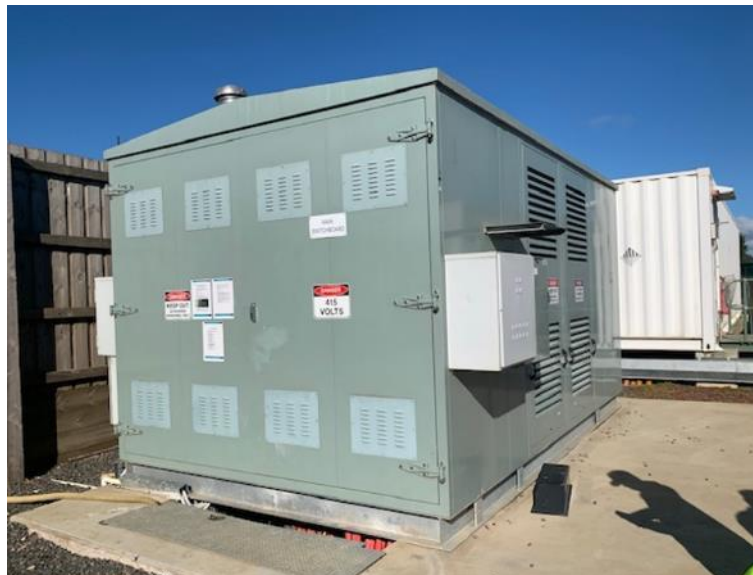
Figure 25: Main switchboard - LV Switchboard with transformer (kiosk)
