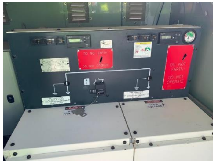
Figure 23: HV Ring Main Unit (RMU)
