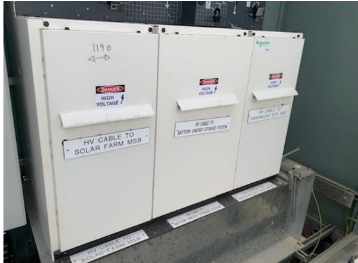
Figure 24: HV cables connection point
