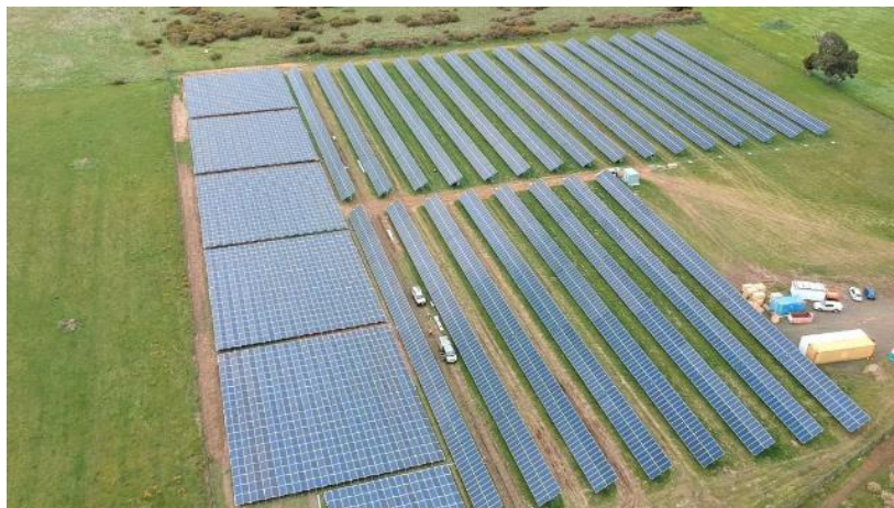
Figure 1: Ariel view of completed solar array.
