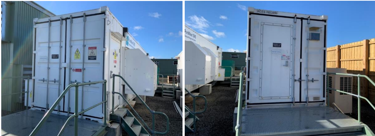
Figure 22: Purewave S&C 2MW/2MWh BESS
