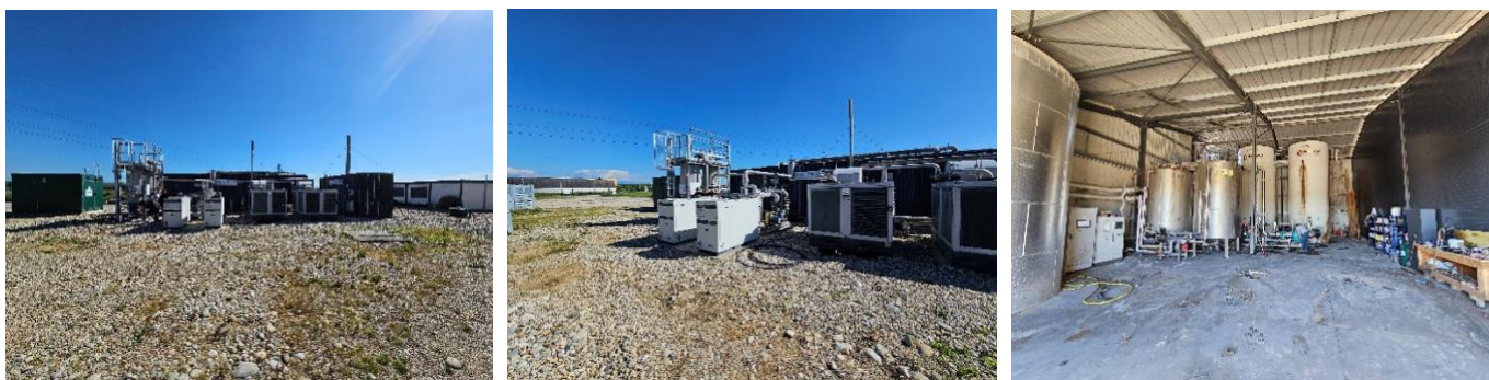
Figure 9. Biomethane Facility at Food Waste Receiving Facility.
