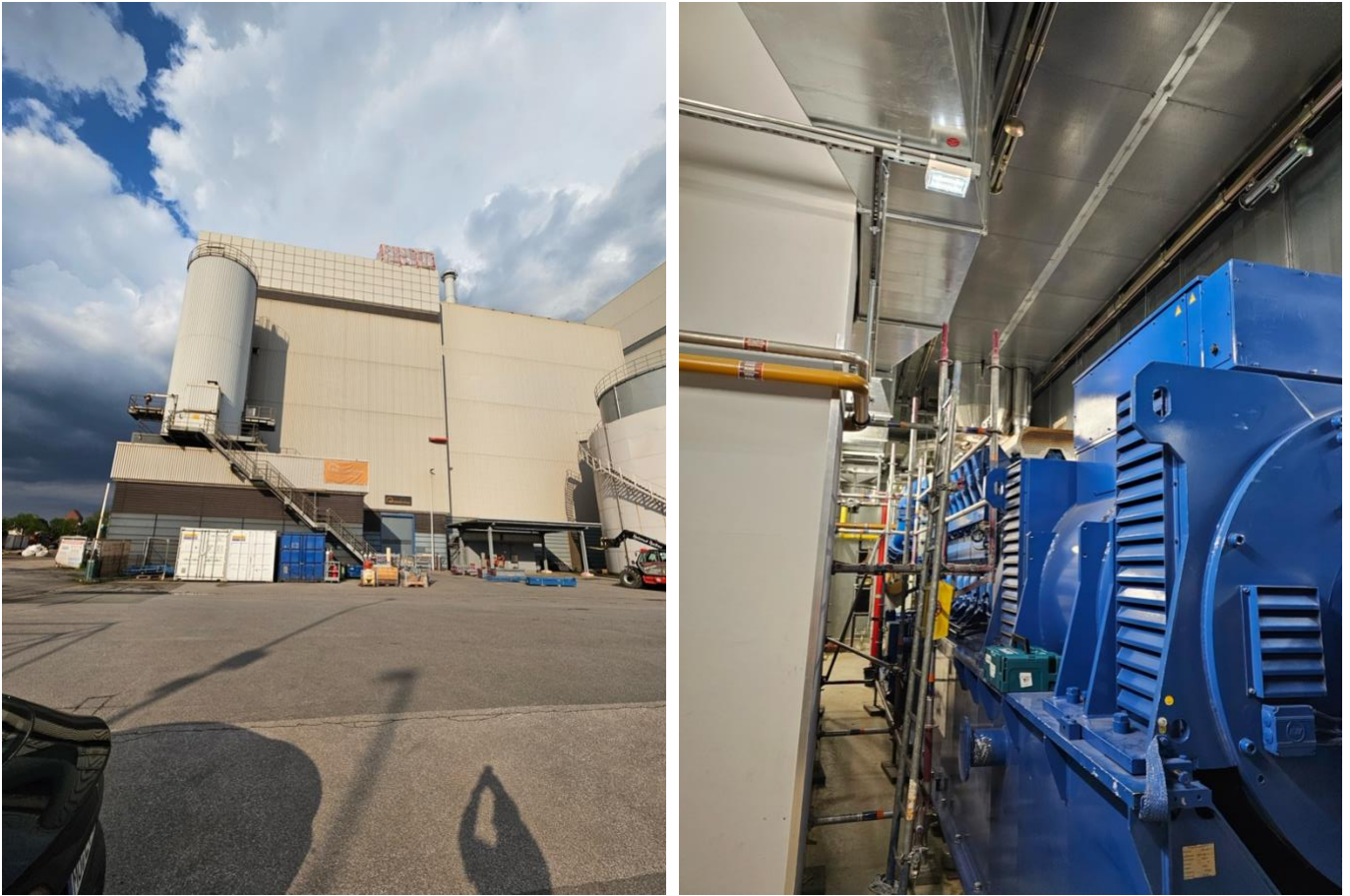
Figure 5. Peaking Cogeneration Plant Duisburg, Germany.
