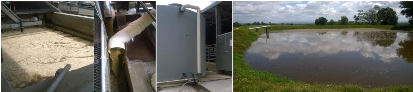
Stabilising settling save-all effluent before pumping to farm
