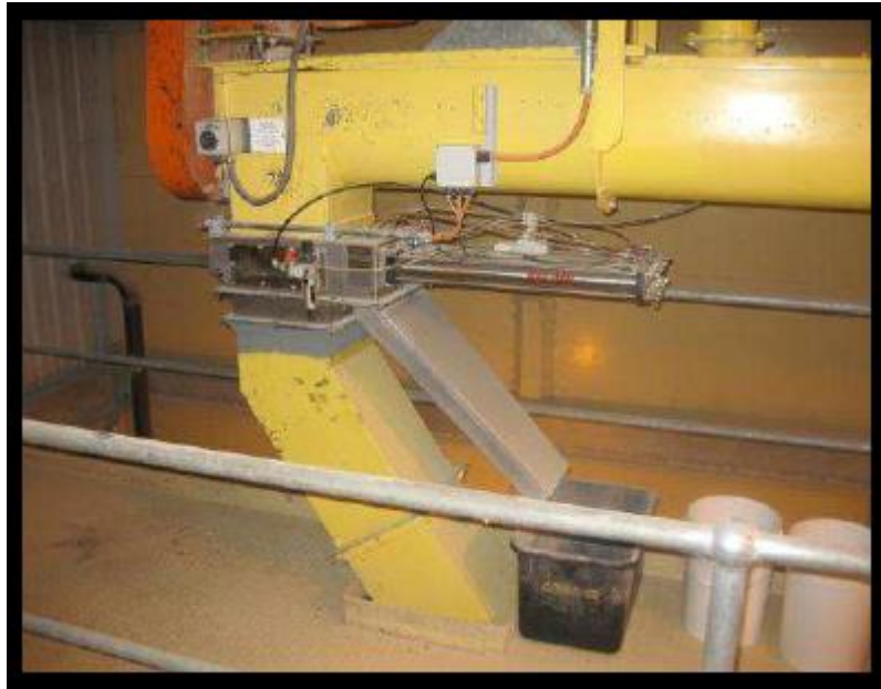
Figure 17: MAGRAM installed in situ.
