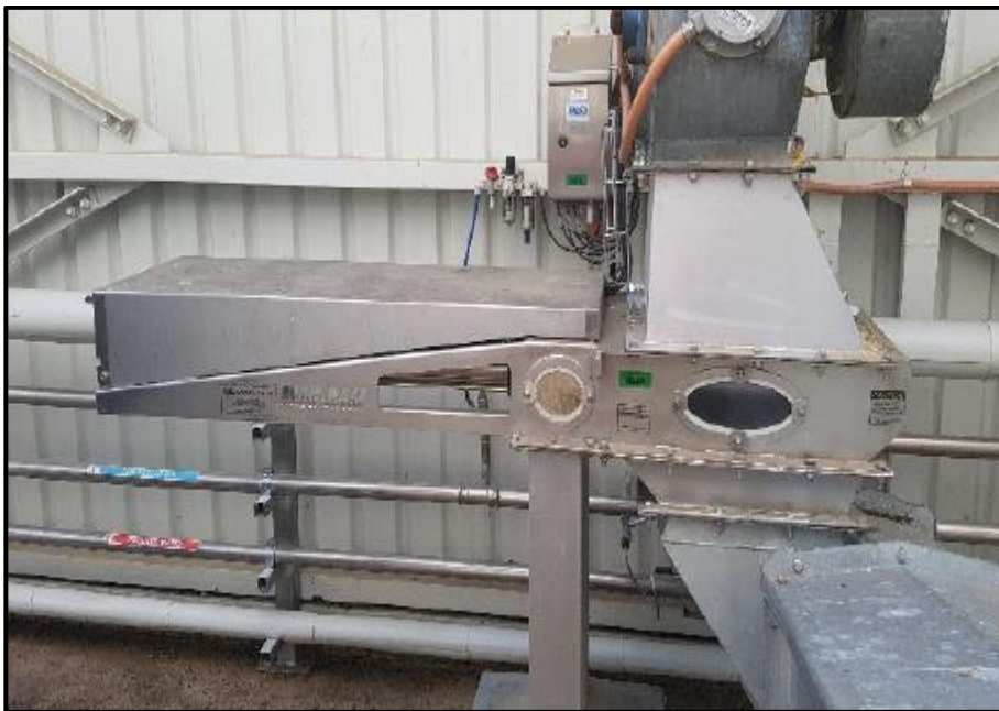
Figure 21: MAGRAM RE80 self-cleaning pneumatic separator installed in situ.
