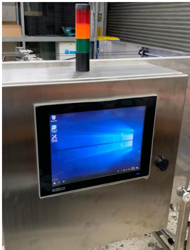
Figure 10: RFID Tunnel and conveyor – User display and light stack
