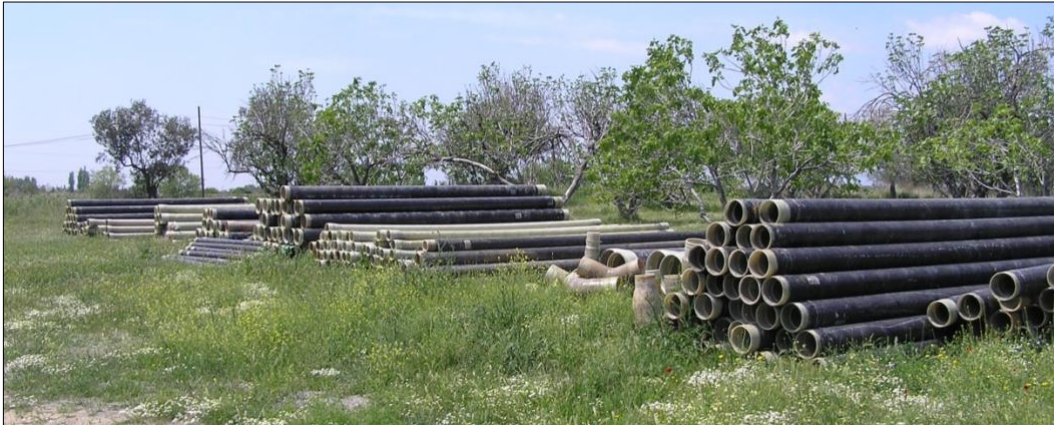
Figure 33: Lengths of casing ready to be emplaced in a geothermal bore in Turkey, 2005
