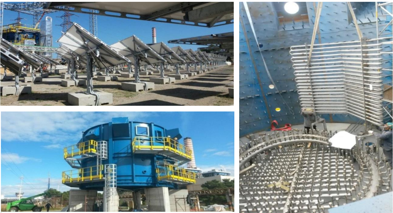
Figure 13: Magaldi STEM Pilot Plant, Italy
