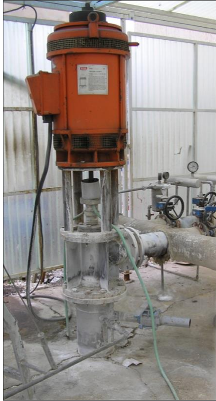
Figure 35: The headworks of a geothermal bore in Turkey, capped with a line-shaft pump motor, 2005
