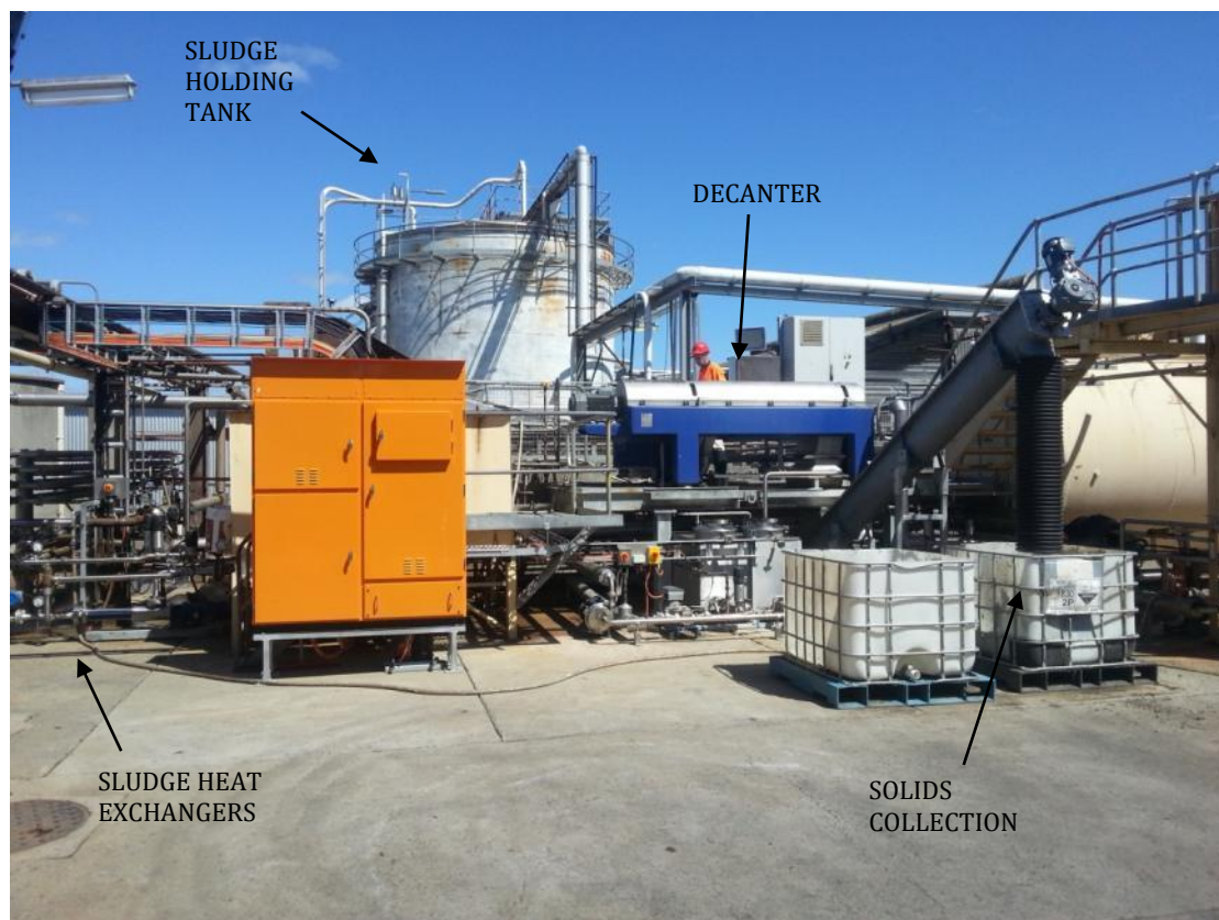
Figure 8. Longford three-way decanter installation
