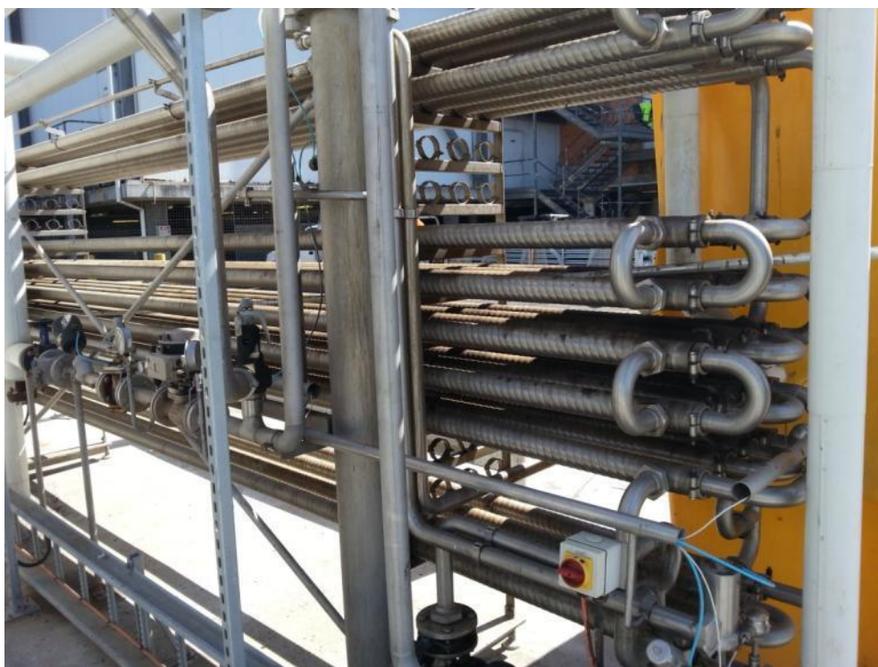
Figure 11. Decanter feed heat exchangers
