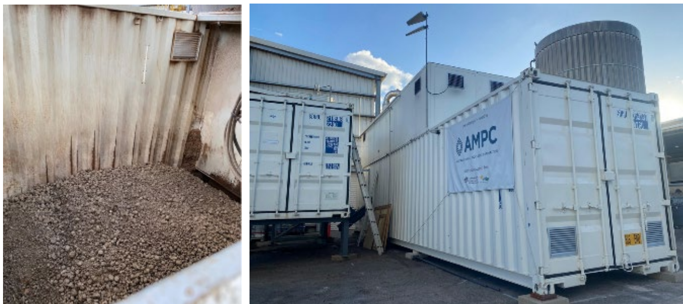
Pellets loaded into the 20' fuel hopper. 20' fuel hopper (left) and 40' containerised boiler (right).
