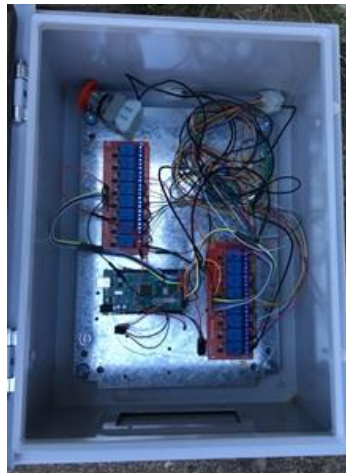
Figure 13. Electrical and control systems.
