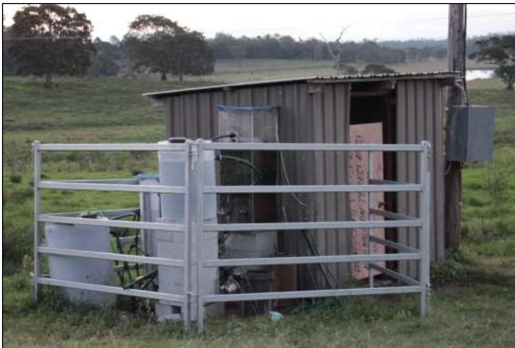
Figure 10: Struvite crystallisation plant installed at Site B to recover phosphorous from anaerobic lagoon effluent
