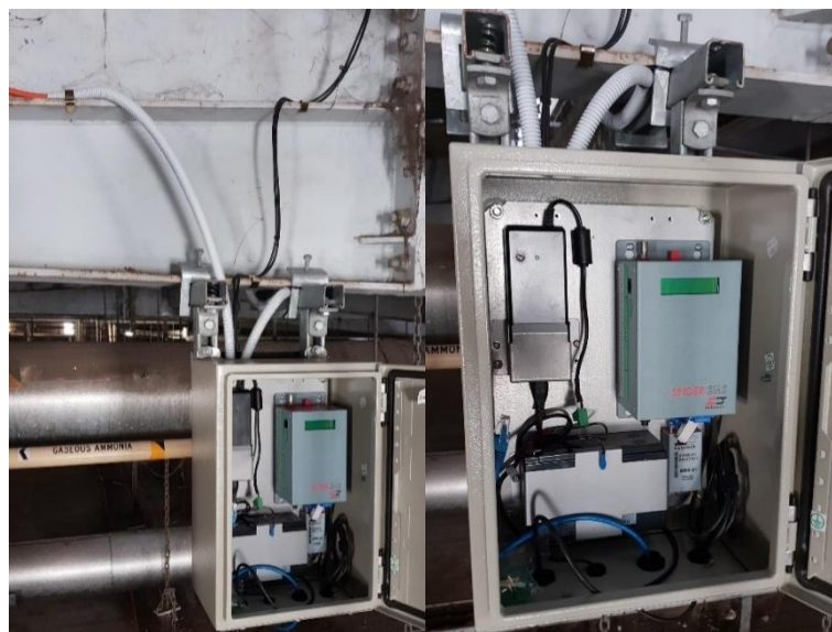
Figure 7: Spider AMR system to transmit water meter data. Source OBEX
