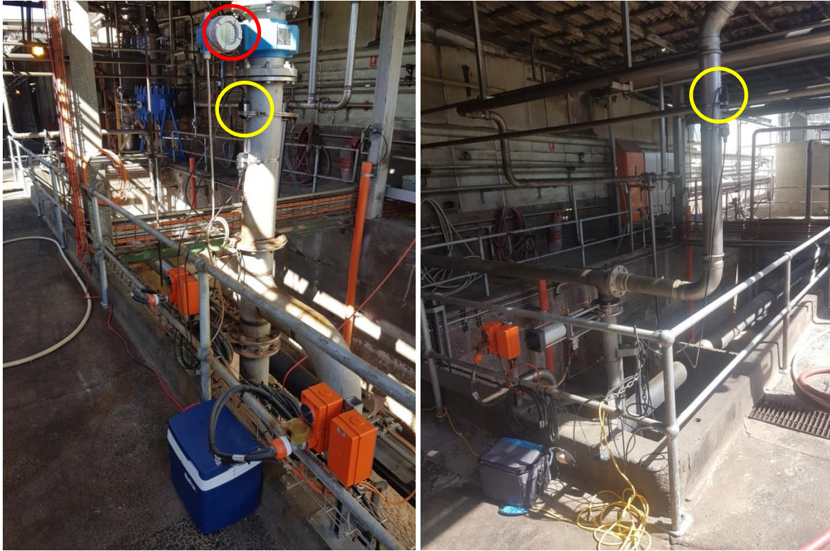
Figure 1: Ultrasonic flowmeters placed on saveall south waste stream (F5) (left) and saveall north waste stream (F9) (right) (yellow circles). Fixed on-site electromagnetic flowmeter on F5 (red circle). See figure 2 for flow metering locations.
