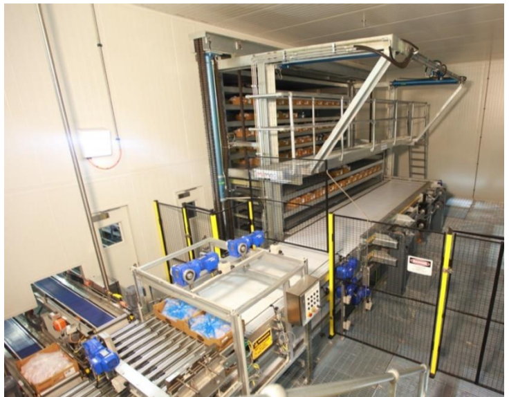
IMAGE 13 – AUTOMATED BLAST FREEZER
