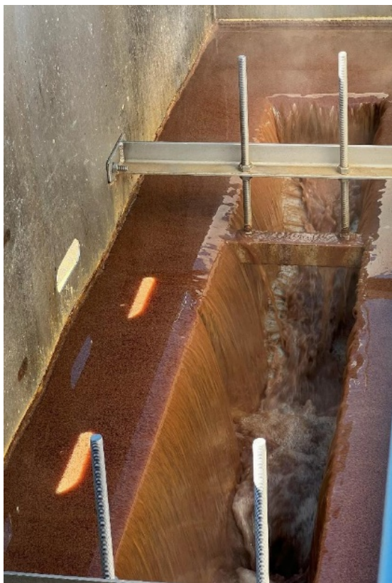
Figure 10. Flocs were in the final clarified water stage of the DAF.
