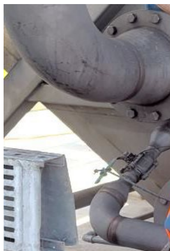
Figure 30. V517 ball valve installed at the end of the saturated water pipe.
