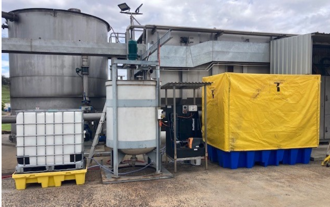
Figure 5. Dosing system configuration. From left to right: neat polymer IBC, polymer tank, make-down skid and Tanfloc IBC bunding. In the background, the pre-DAF tank appears on the left, followed by the DAF on the right-hand side.
