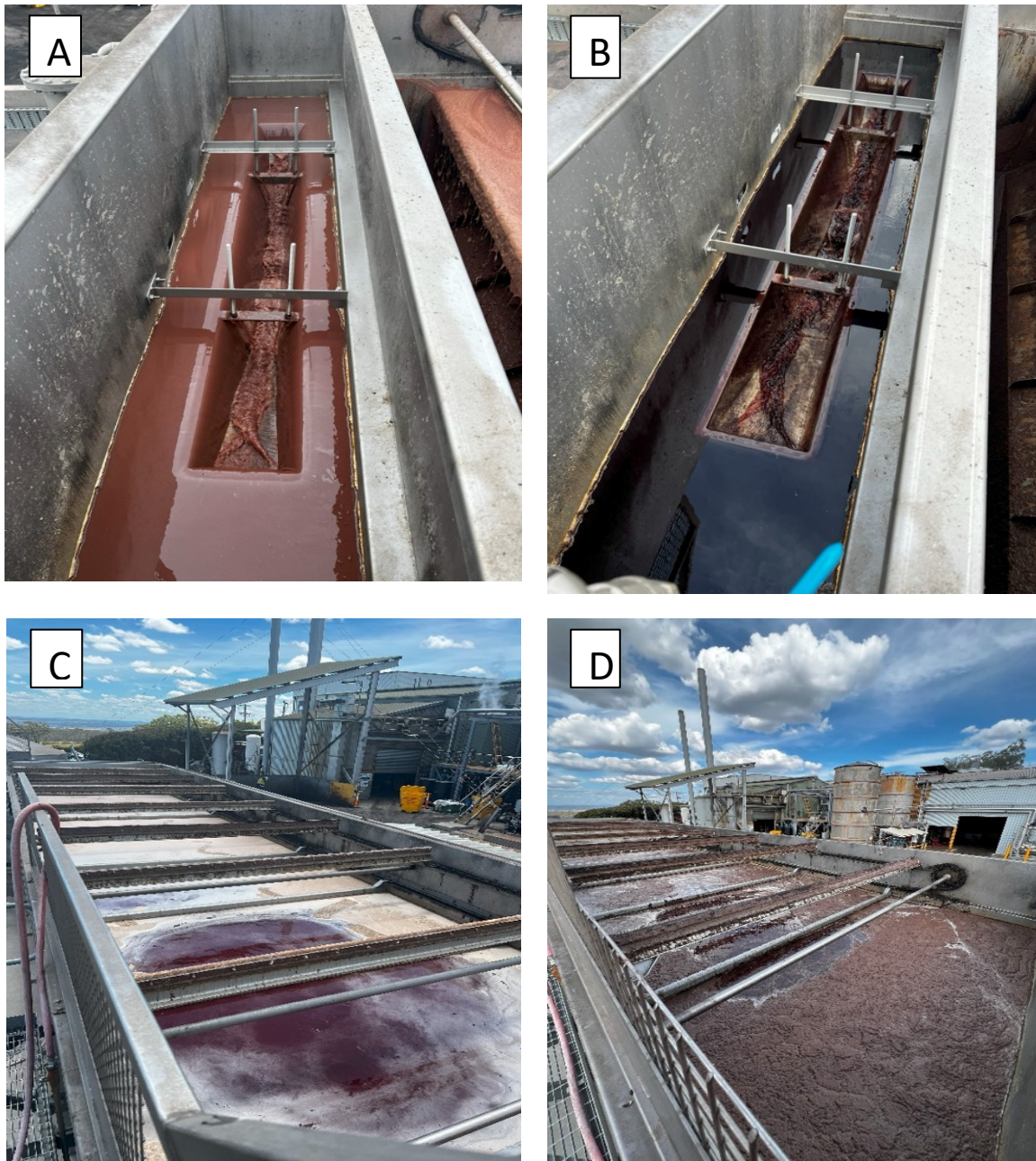
Figure 12. Clarification chamber before chemical dosing (A). Clarification chamber after chemical dosing (B). DAF reservoir before chemical dosing (C). DAF reservoir after chemical dosing (D).
