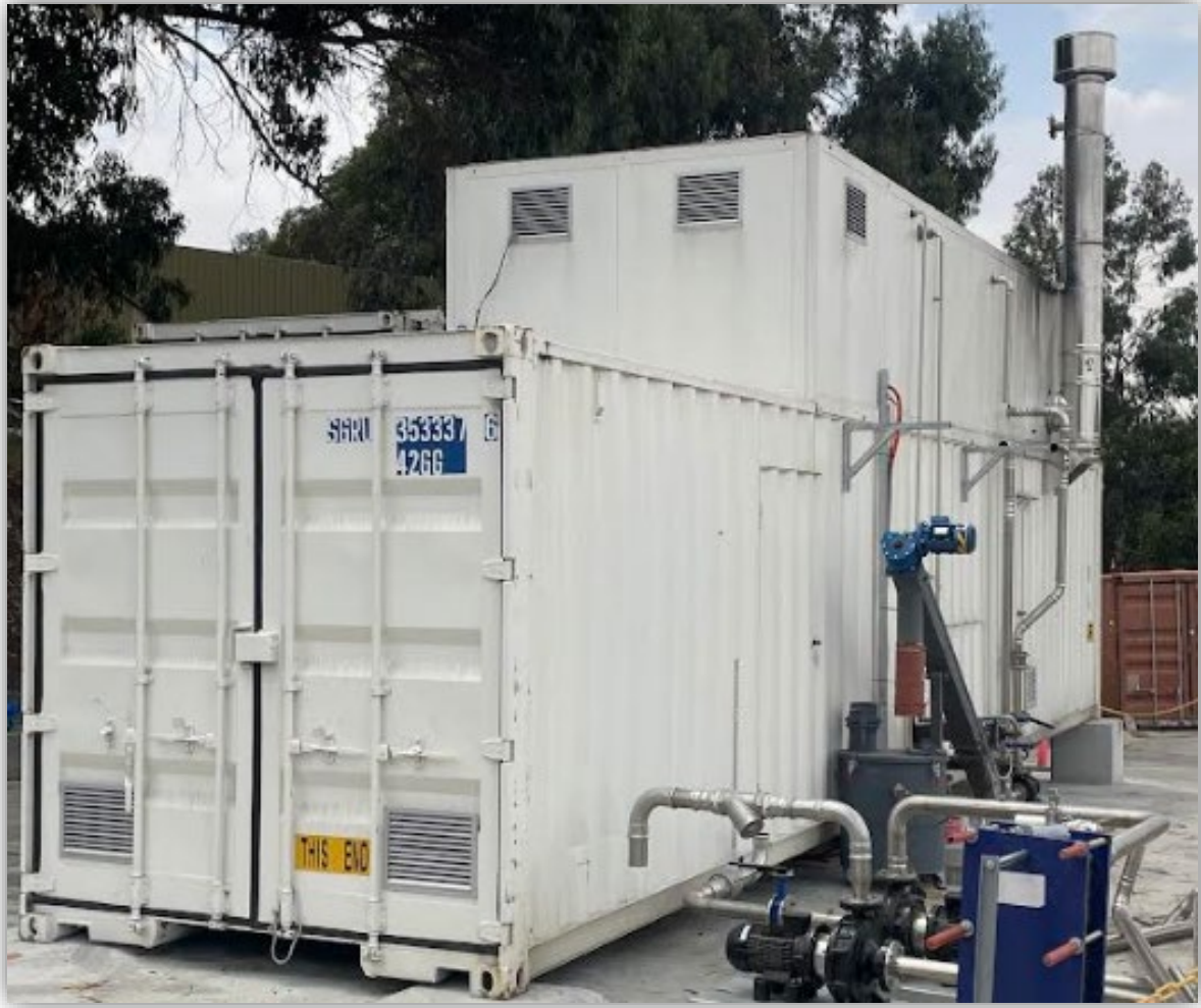
Figure 2: Biomass Pilot installed in SA.
