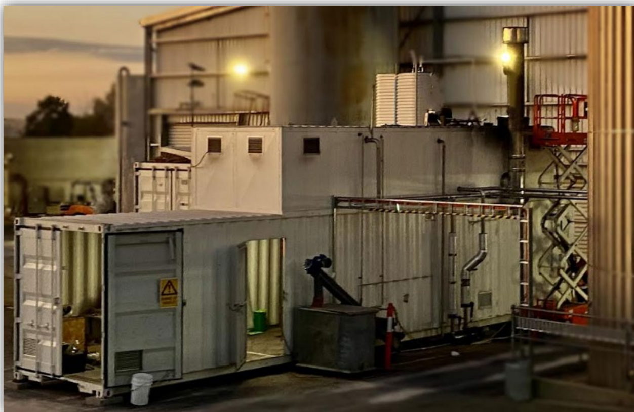
Figure 1: Biomass Pilot installed in NSW. The 40' containerised boiler is in the front of the image, with the 20' fuel hopper located behind.
