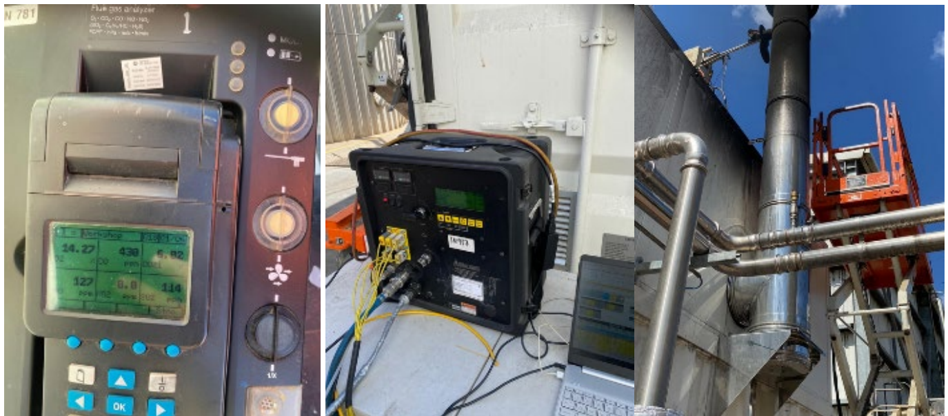
Figure 11: Left to right: real time emissions data readouts, data logger and HMI, in-stack probe using the 110mm port at NSW pilot location.
