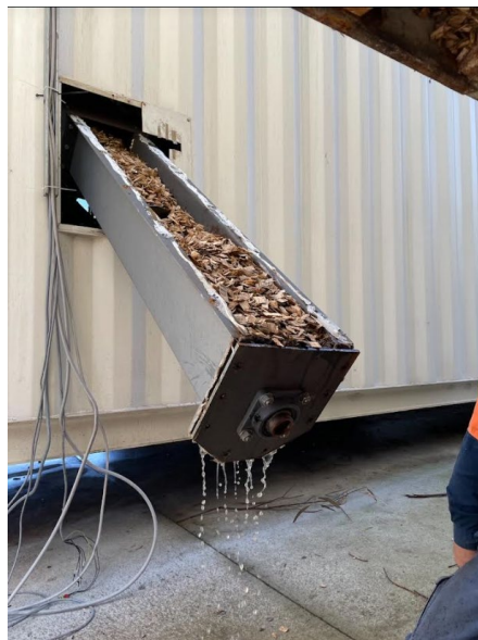
Photo of final demobilisation showing water draining out of auger connecting the 20' fuel storage with the 40' mani boiler container.
