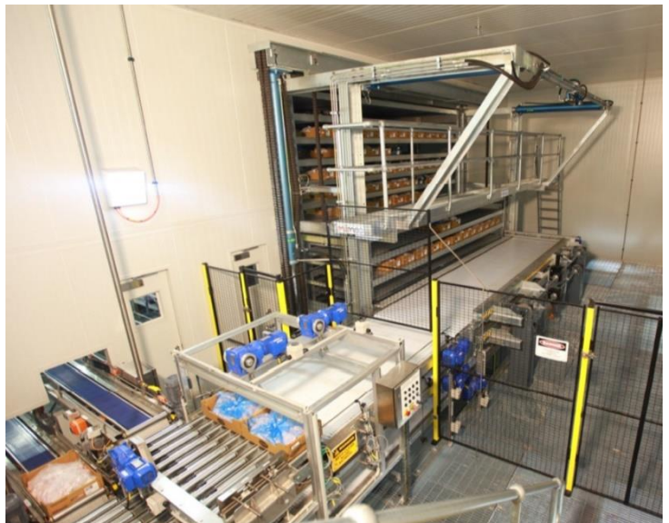
IMAGE 13 – AUTOMATED BLAST FREEZER
