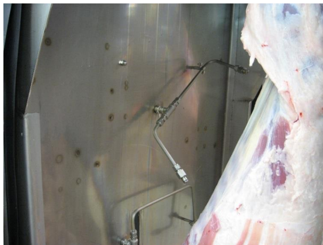
Image 4: Hot water sprays turn on when cabinet doors close to assist in controlling hot water and aerosols.
