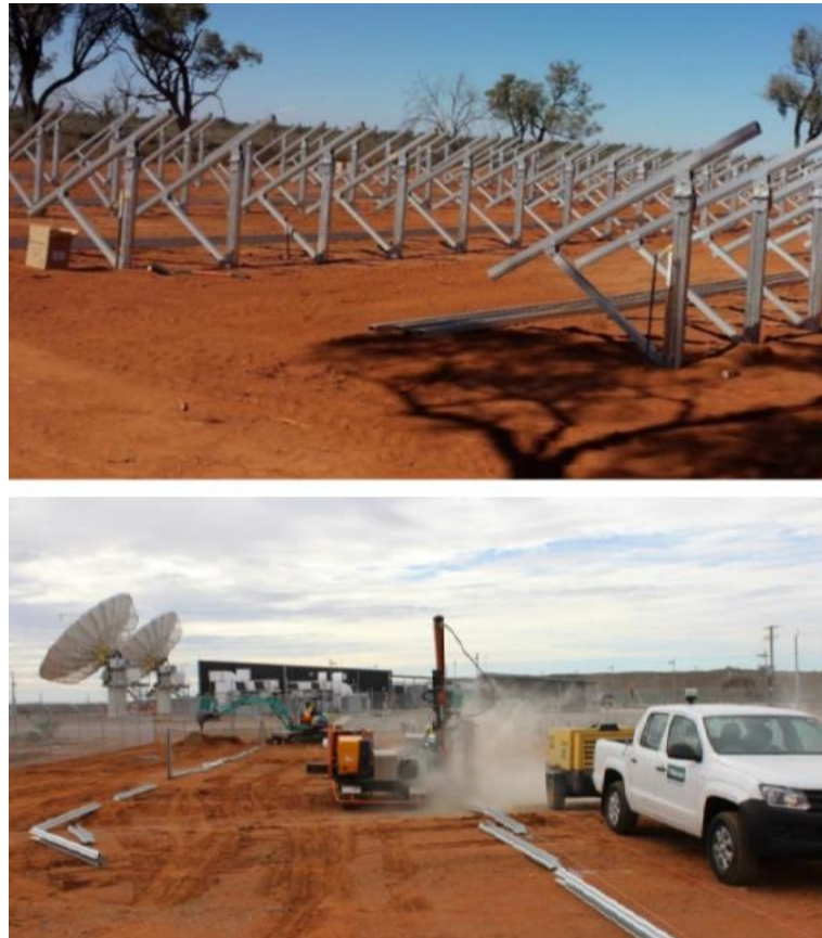
Figure 15: Solgen ground mounted system at NBN Broken Hill.
