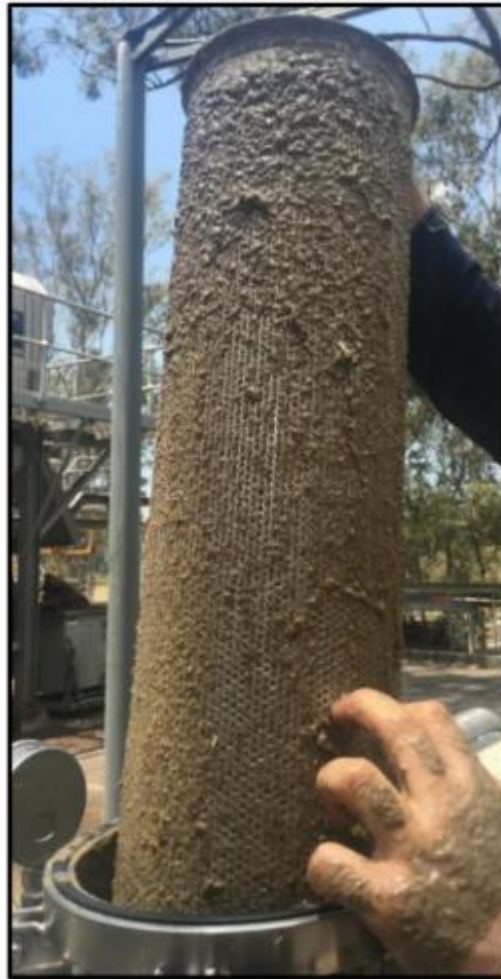
Figure 10: DAF float clogging the pump filter during trial.
