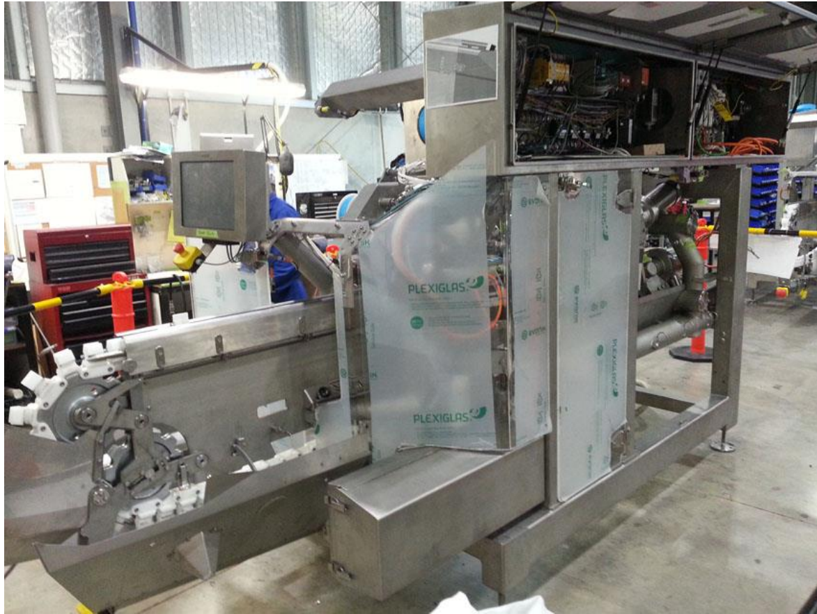
Figure 3-4 - Control cabinet and reticulation
