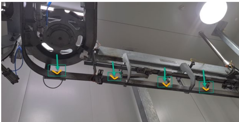
Figure 16: Annotated Infeed rail showing the grooves in the rail to better secure the skid when moving along the rail.
