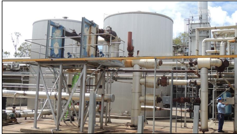
Heat Storage and Piping
