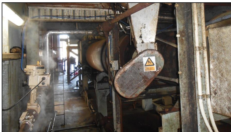
Obvious and costly steam leaks from piping
