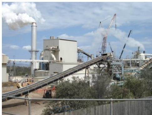
Figure 3: Tablelands Sugar Mill Bagasse-fired Steam Generator
